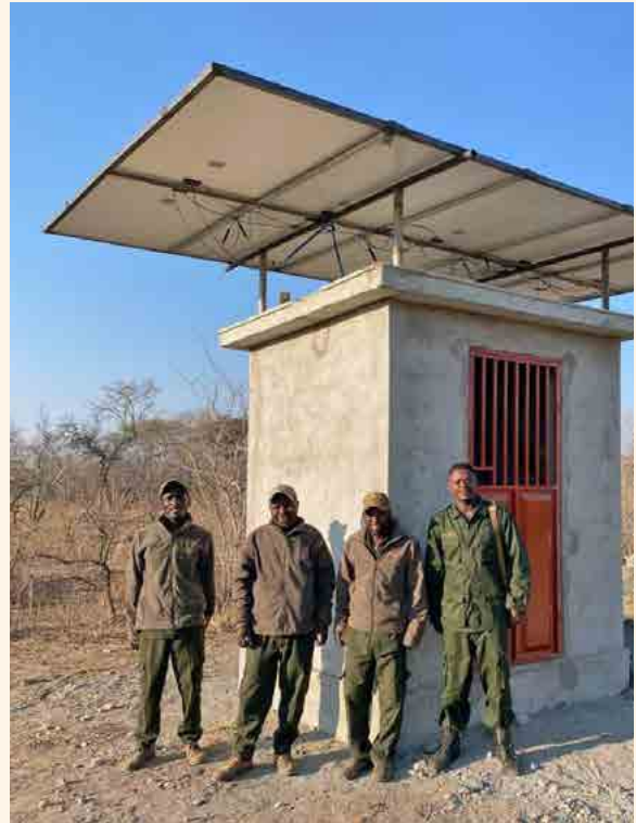
Solar panels for powering the water pump.
