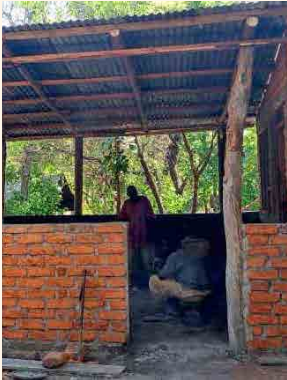
Staff canteen under construction at Fish Eagle Camp. Rain proof and comfortable with a separate room for storing food safely.
