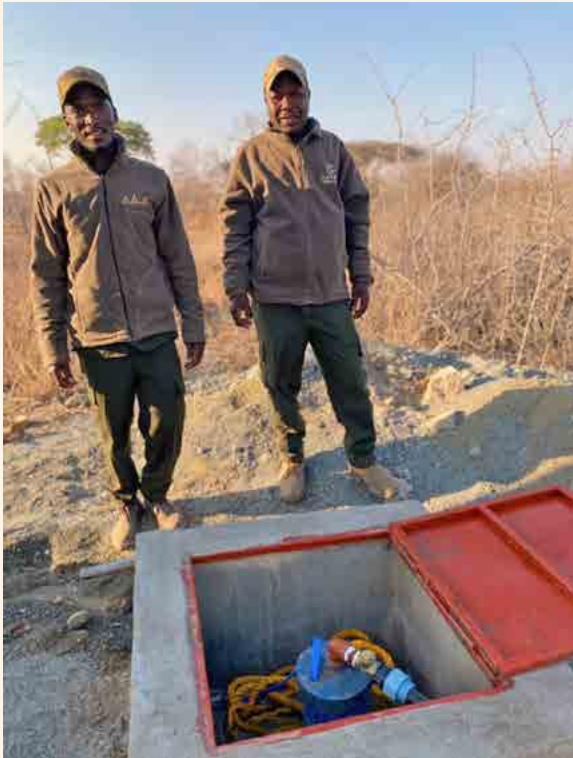
Borehole site and pump location.
